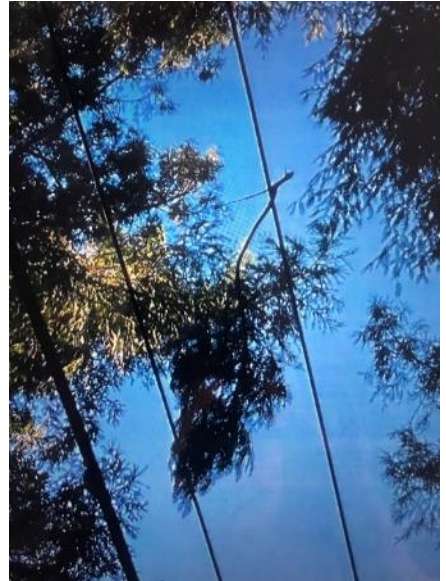
Figure 15: Image of Vegetation Hazard in Santa Clara County - Branch on Conductor
