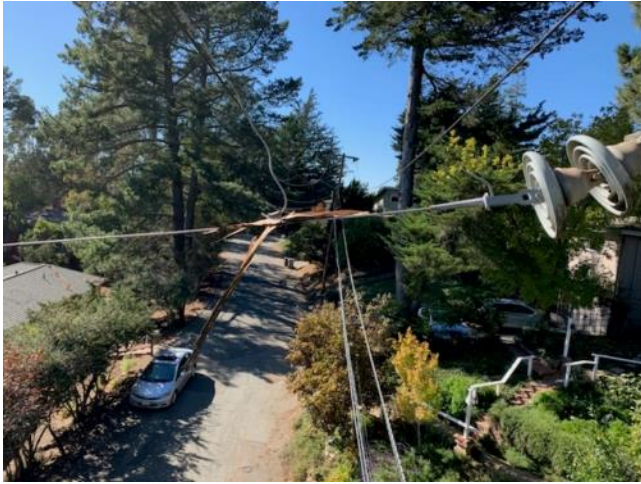
Figure 19: Image of Vegetation Hazard in Alameda County – Bark Found on Primary
