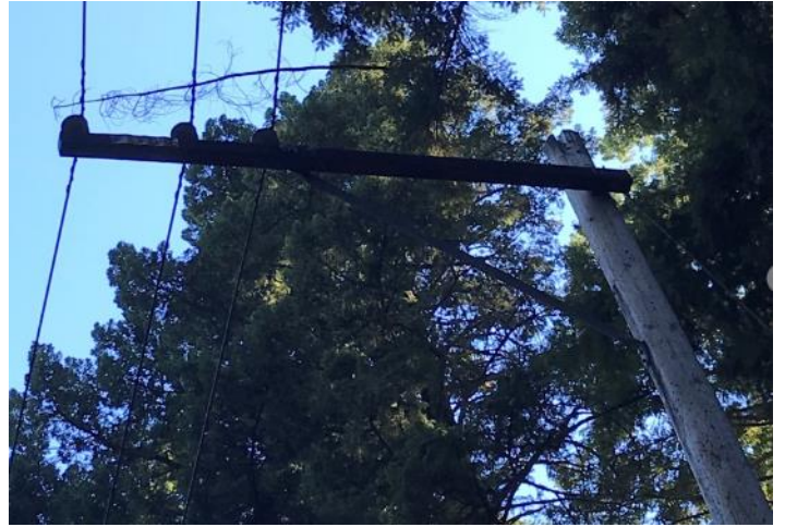
Figure 20: Image of Vegetation Hazard in Santa Cruz County – branch across all 3 phases of 12kV primary circuit
