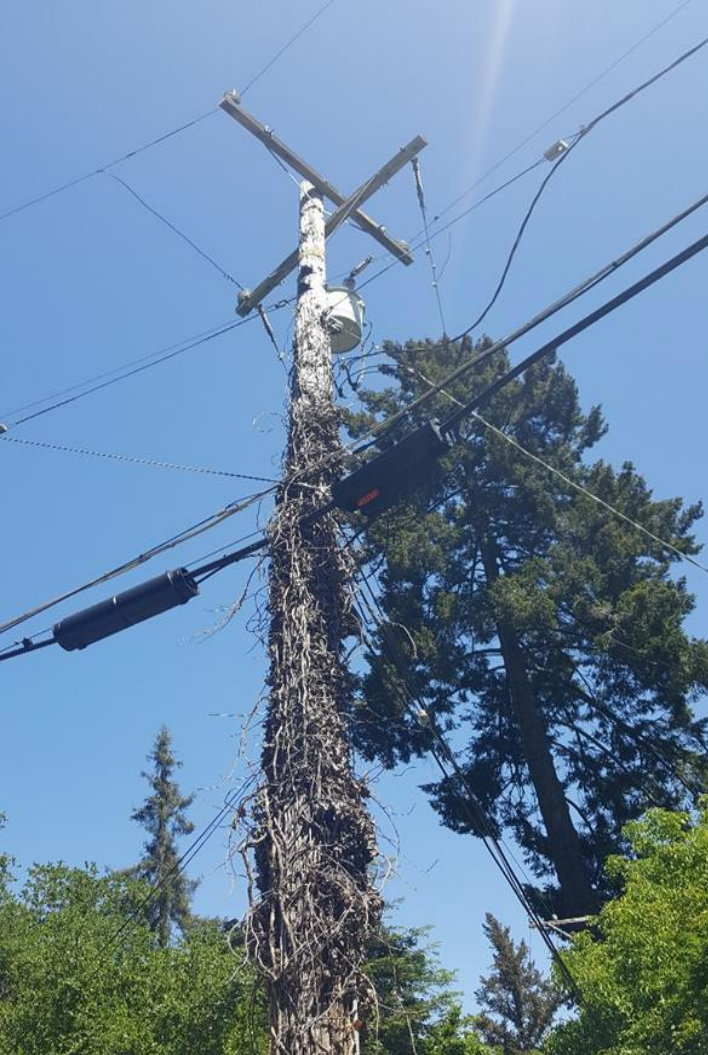
Photo: Tier 3 High Wildfire Danger Area, Los Gatos, CA, Utility pole wrapped with dead vegetation, Photo by Prof. Catherine Sandoval, May 2019
