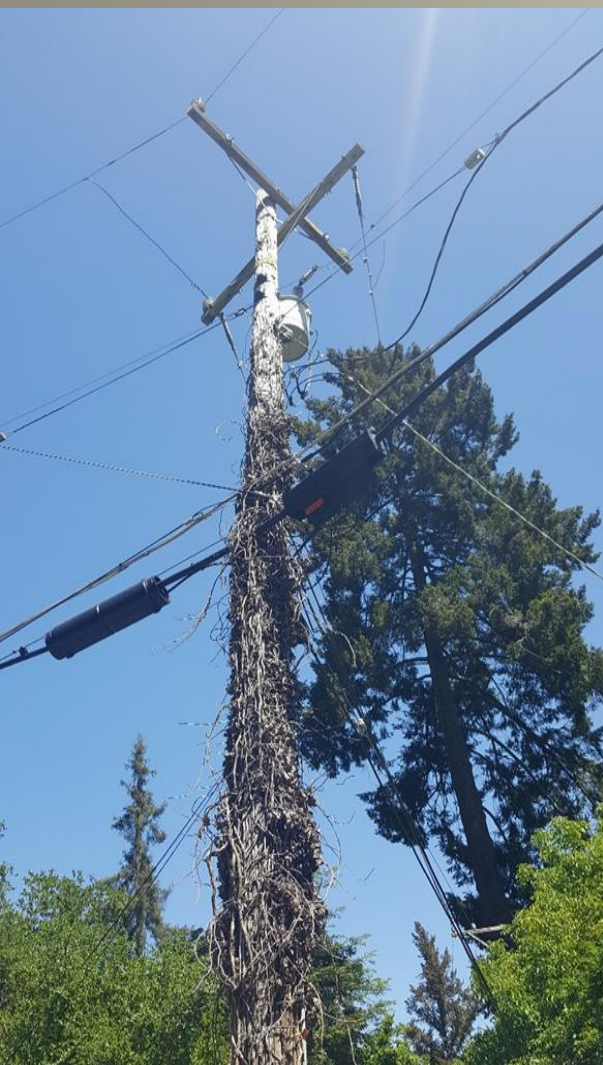
Photo: Tier 3 High Wildfire Danger Area, Los Gatos, CA, Utility pole wrapped with dead vegetation, Photo by Prof. Catherine Sandoval, May 2019
