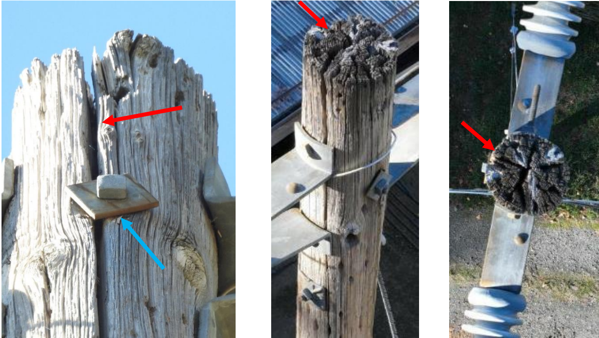
Figure 8: Left: ISM ground photo taken showing hardware (blue arrow) through split (red arrow) in pole; Middle: PG&E Drone Photo from opposite side of pole. Red arrow shows location of the split on the opposite side of pole. Right: PG&E Drone photo showing top view of pole. The red arrow shows the location of the split. PG&E did not have an aerial photo of the side of the pole which showed the split in the ISM photo.
