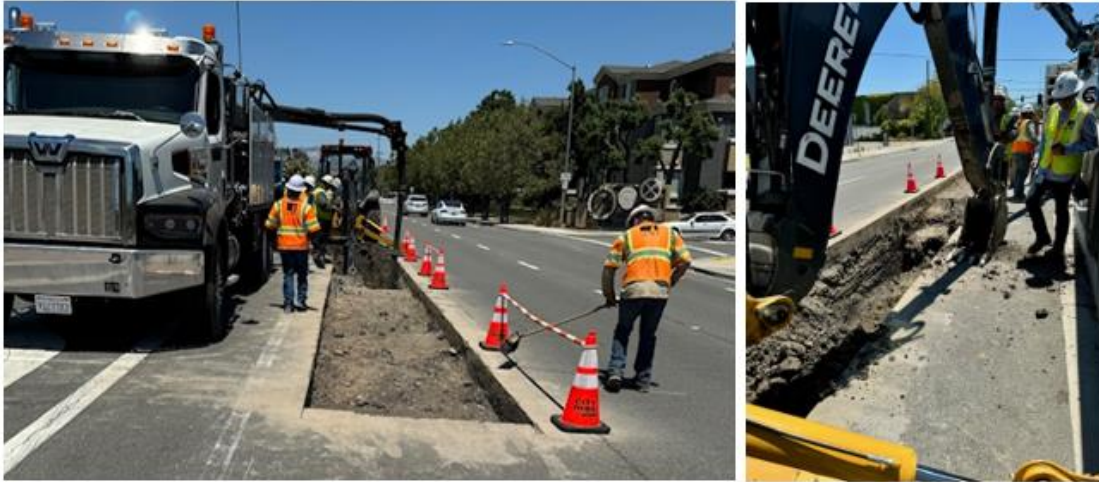
Figure 18: Excavation by backhoe and vacuum truck to expose the steel pipe and plastic casing
