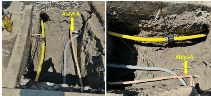
Figure 17: Excavation with the new 2-inch distribution PE pipe, older Aldyl-A pipe, and other utilities
