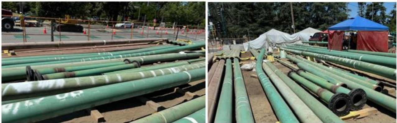
Figure 19: Temporary pipe yard representing hundreds of feet of 10-inch steel pipe for transmission pipeline relocation
