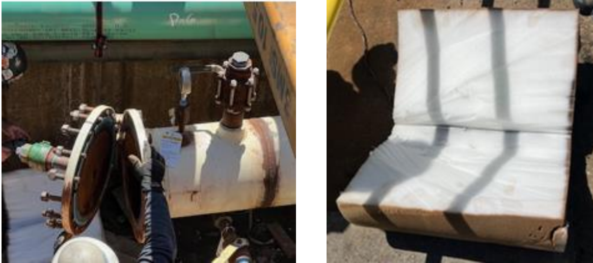
Figure 21: 12-inch foam pig being examined (right) after removal from receiver (left), with visible dry foam and pipe residue.
