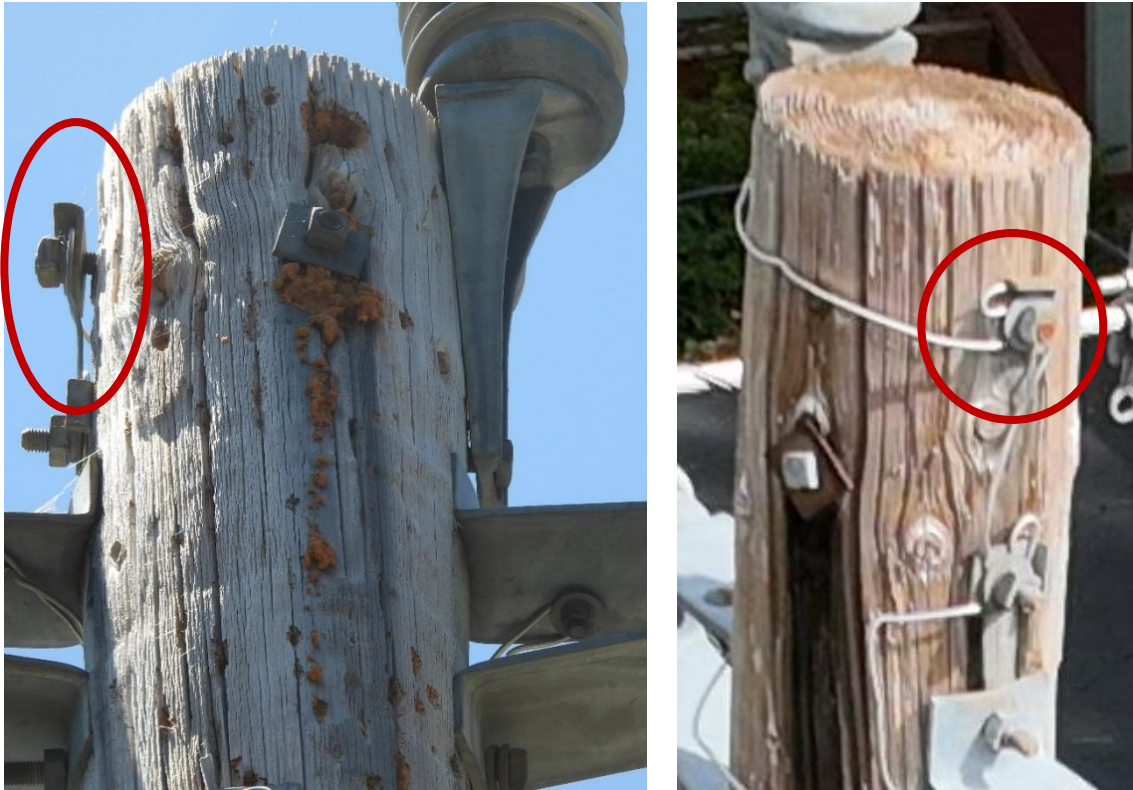
Figure 6: Left: Photo taken by the ISM of loose hardware; Right: Drone photo of the loose hardware identified in the left photo.
