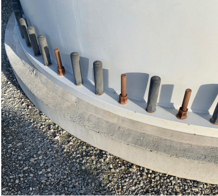
Figure 10. Missing bolt covers at tower base of WTG F4.
