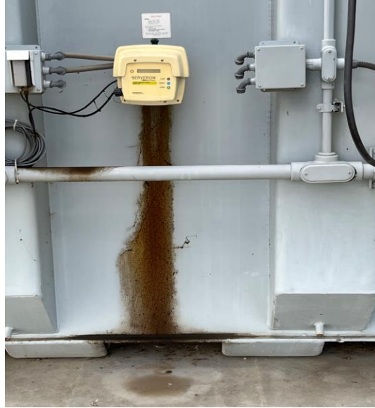
Figure 5. Oil leak from Serveron valve.
