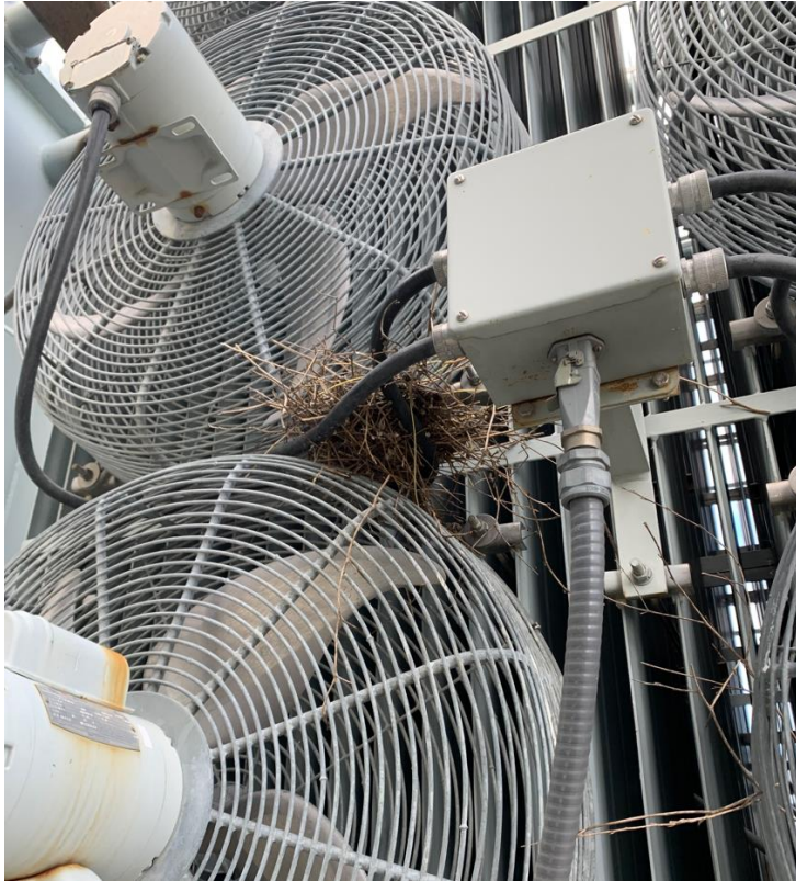
Figure 9. Bird nest near radiator fans.
