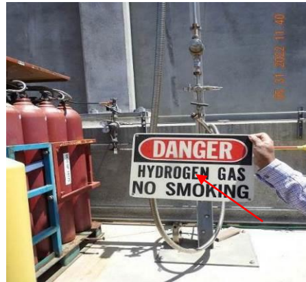
Danger sign not properly attached
