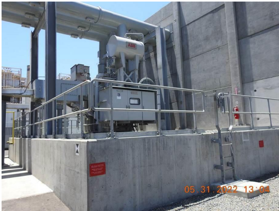
Missing High Voltage sign
