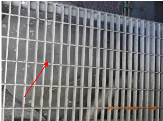
Missing Confined Space Sign
