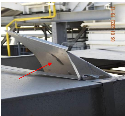
Broken cover of Cable Tray
