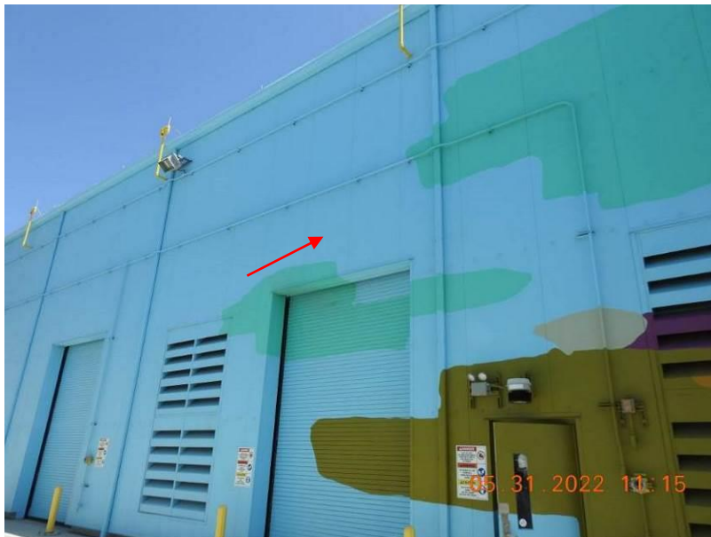
Missing NFPA sign (fire diamond)
