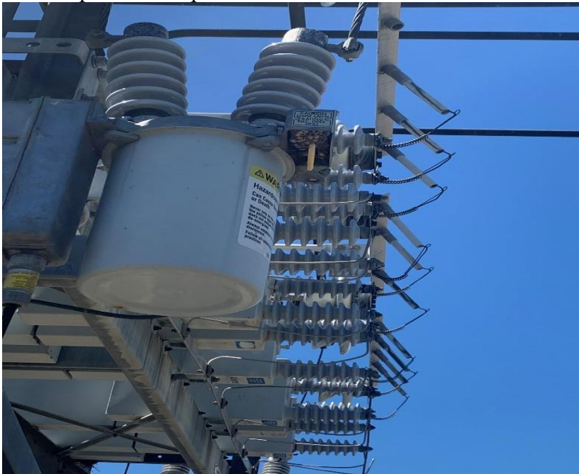
13.3 Wasp Nest at Capacitor Bank 1C. PG&E Fixed in Field.
