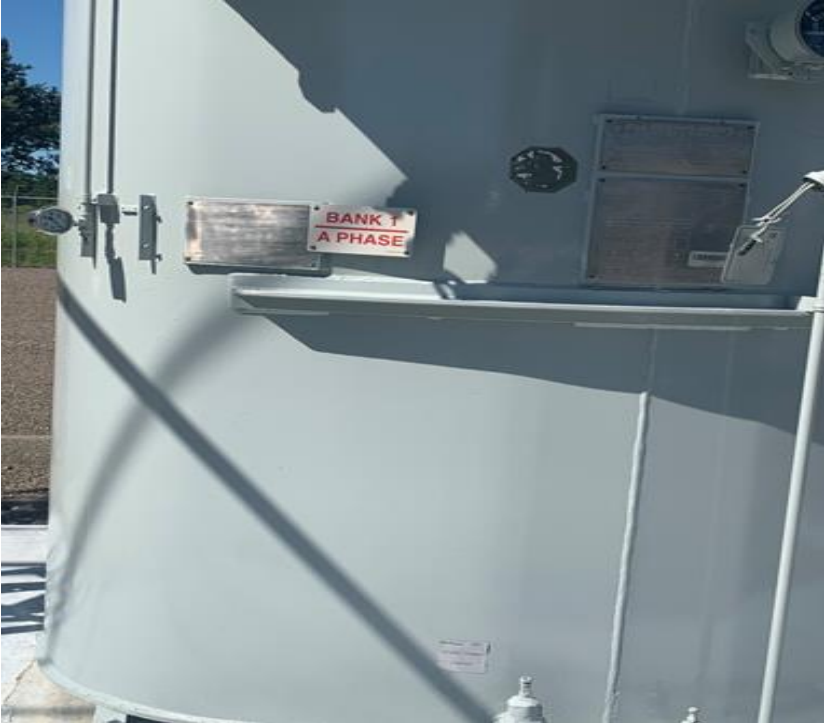
16.4 Transformer Bank Phase A Label For Tank Entry is Damaged
