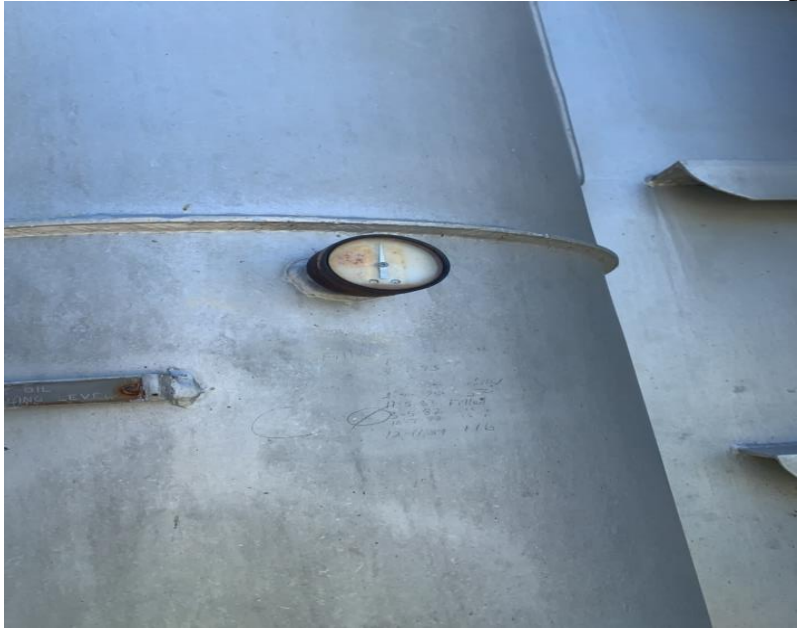
14.3 Transformer Bank 1 Phase C has a Faded Oil Level Gauge
