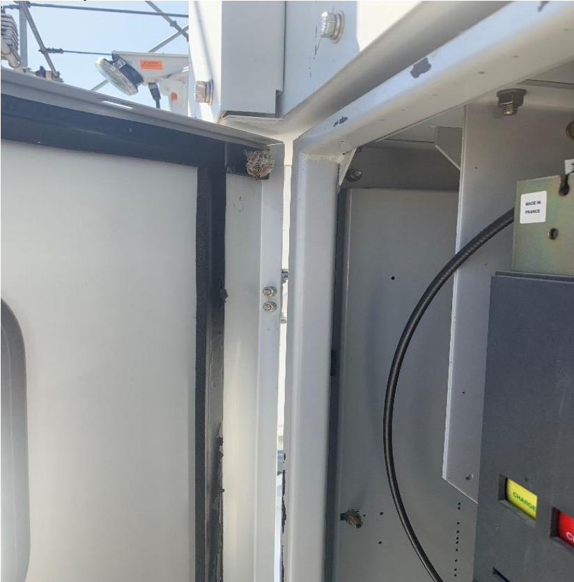
16.3 Wasp Nest Inside Circuit Breaker Cabinet
