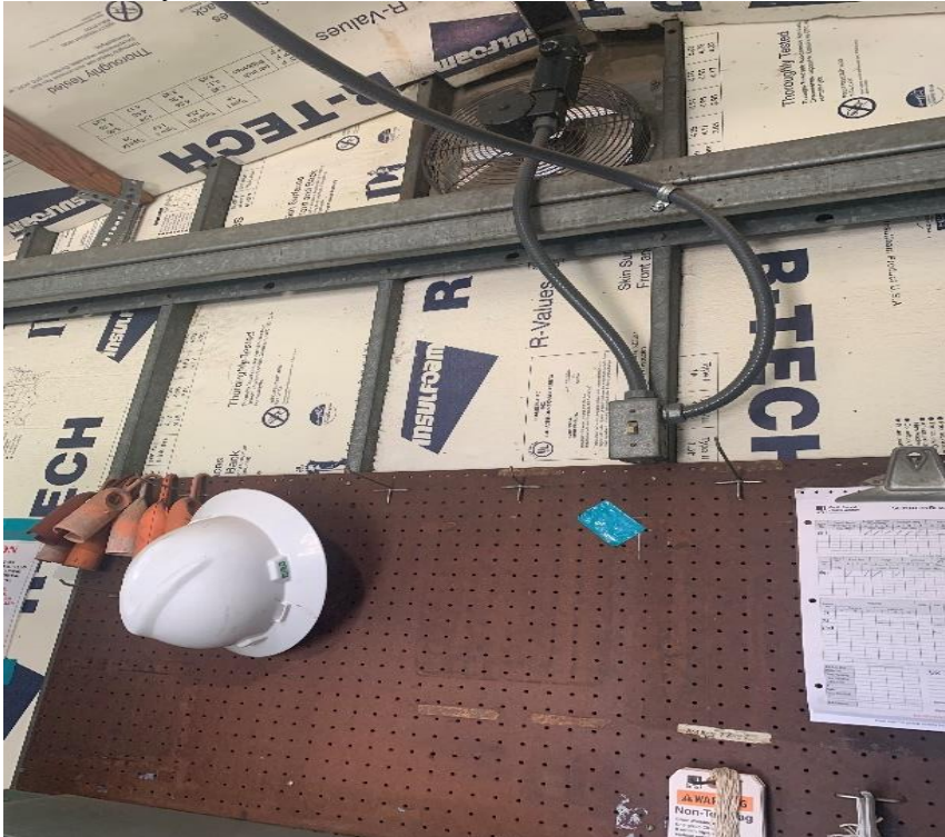
13.5 Battery Room Fan Was Not Working
