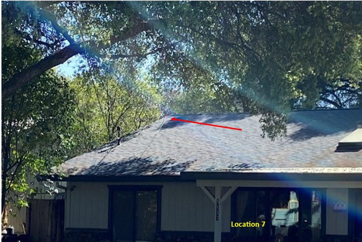
Figure 3: Clearance Issue at Location 7 and 18
