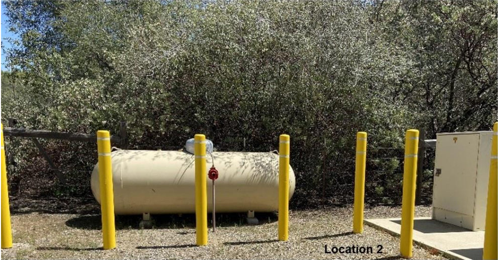
Figure 7: Inadequate labeling at Location 2 and 14
