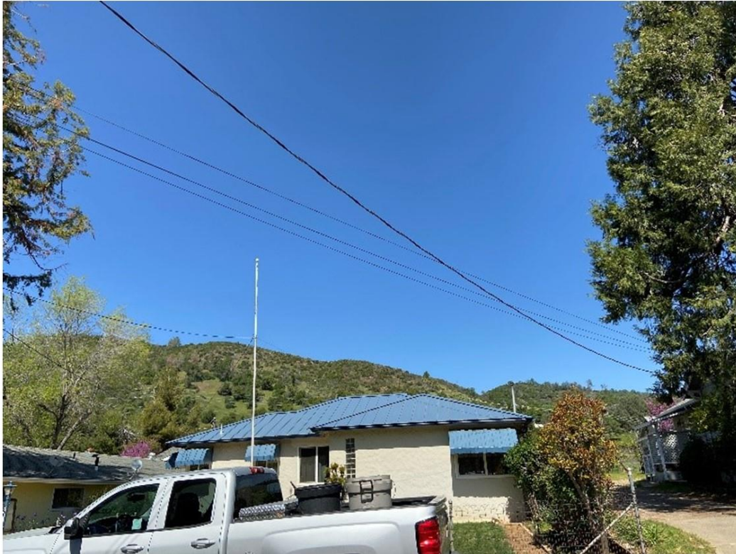
Figure 2: Clearance Issue at Location 10
