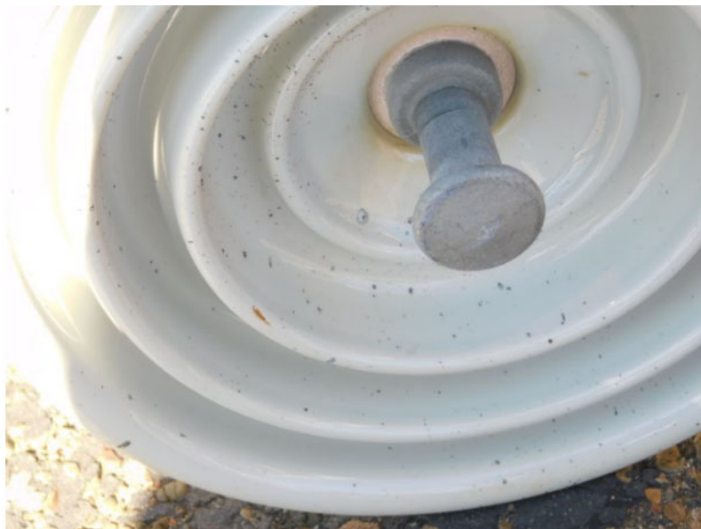
Figure 18: Insulator string that was attached to incident Jumper Cable. The grey spots on the ceramic “skirt” are the arcing residue.
