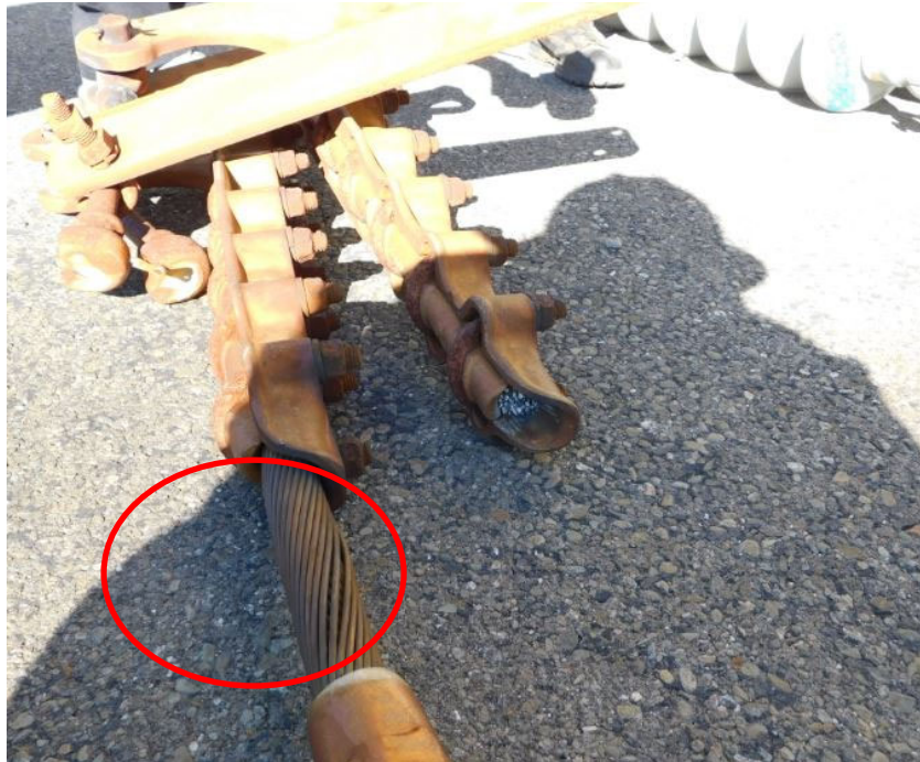
Figure 13: Shoes of the failed jumper cable. Note slight caging on cable that has not failed.
