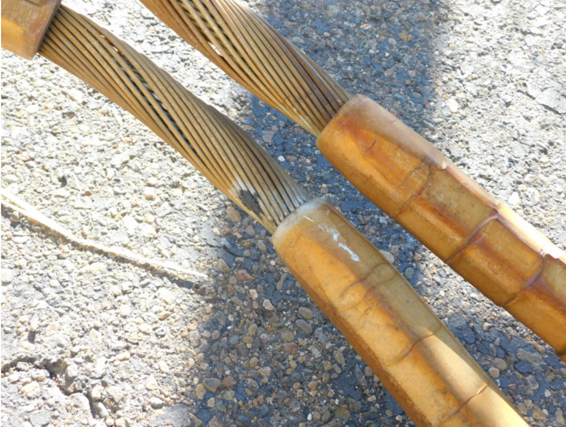
Figure 14: Signs of caging on intact jumper cables removed from the Incident Tower.
