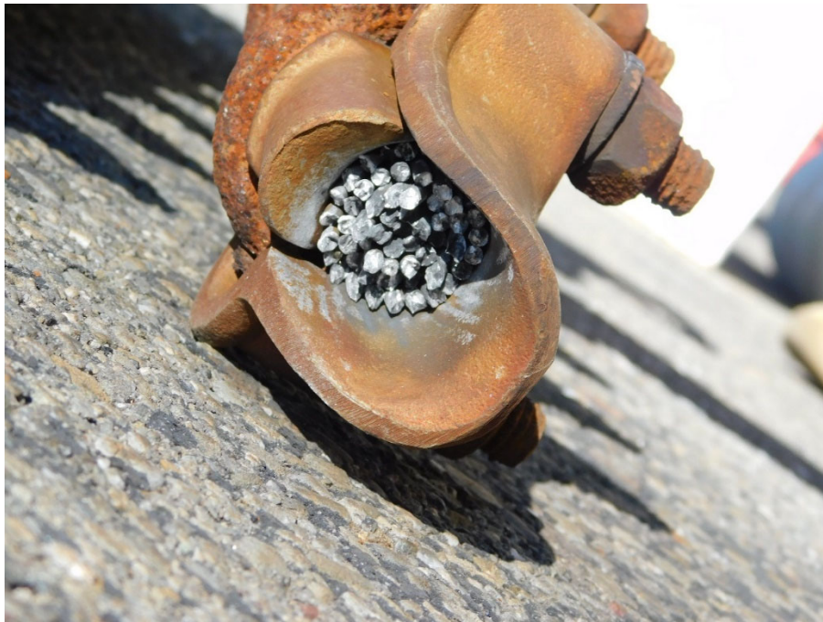
Figure 11: View of the failure point. This segment is still inside the shoe.
