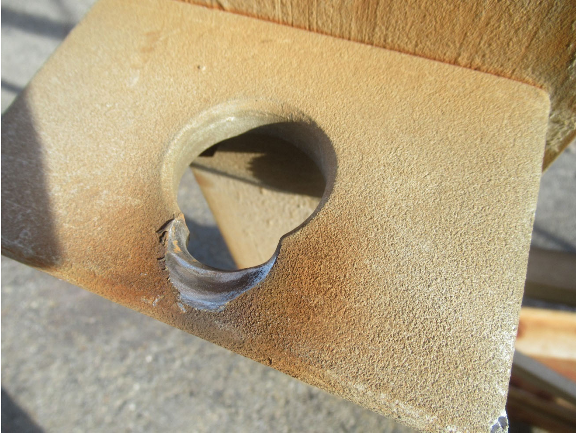
Figure 8: Bolt hole on tower arm collected by PG&E on November 13, 2019.
