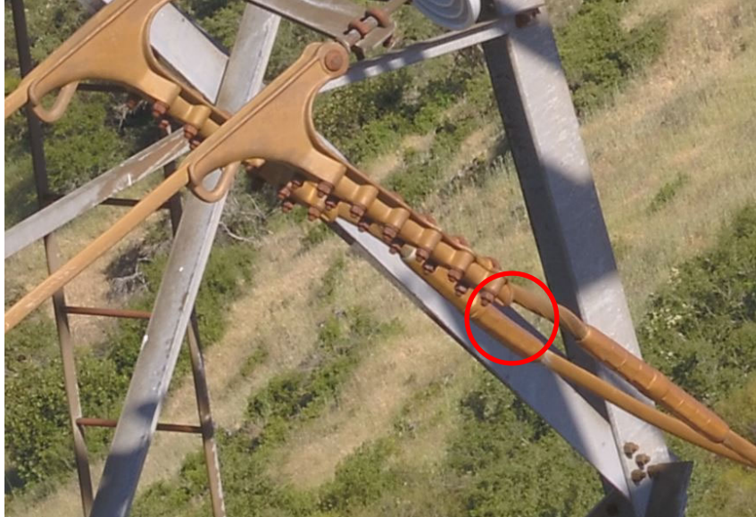
Figure 17: Jumper cable and shoe from May 11, 2019 drone inspection. Note signs of caging/bowing near shoe closer to the camera. 59
