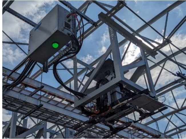
Figure 187. Pantograph Charging System Installed to Serve a Transit Bus Site
