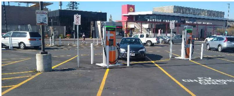
Figure 228. SDG&E Schools and Parks Pilots Example of Already High Access, and Even Higher with Longer Cords
