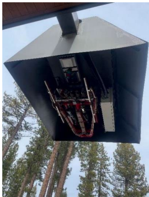
Figure 262. Liberty EV Bus Infrastructure Program Detailed View of Pantograph Mechanism and Protective Cover
